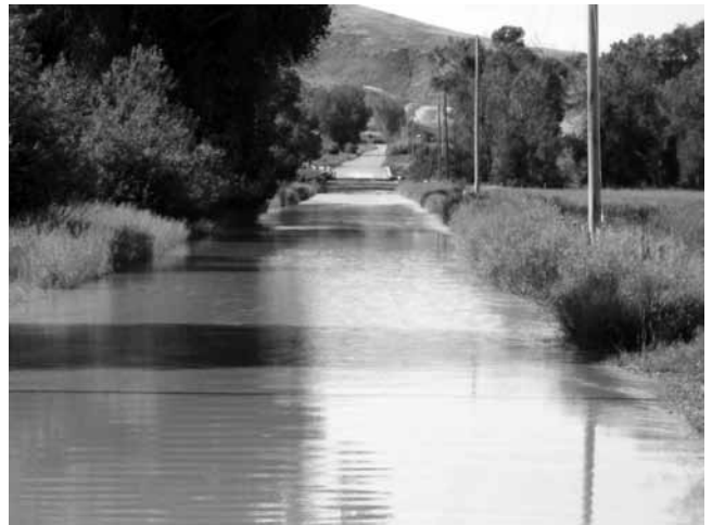
This road is completely under water near Shell.
